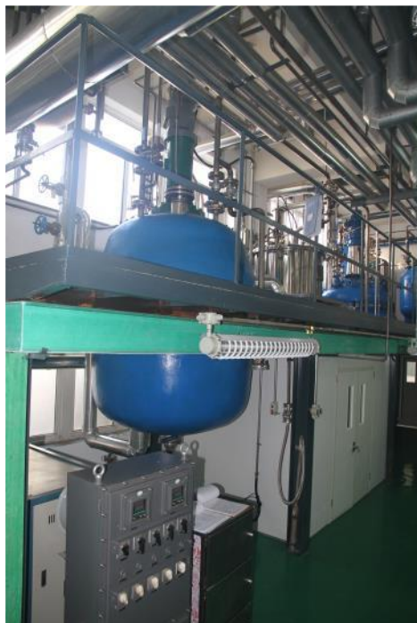
High Temperature Control Panel & Receiving Tank
