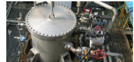
Installed filtration skid system at your site
